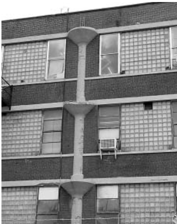
The reinforced-concrete mushroom-column construction of this former RCA Victor factory, built about 1920, is clearly expressed. It now houses the Musée des ondes Émile Berliner that pays tribute to the inventor of the flat recording disk through an impressive collection of phonographs, radio receivers, tape recorders, and television sets. The museum held tours for several SIA groups.
