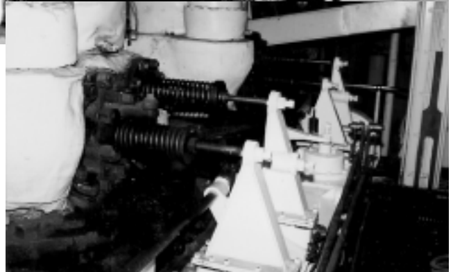
Midsection of the Badger's port engine, between the (upper) high-pressure cylinders and (lower) low-pressure cylinders, showing the bell cranks that operate the steam valves.
